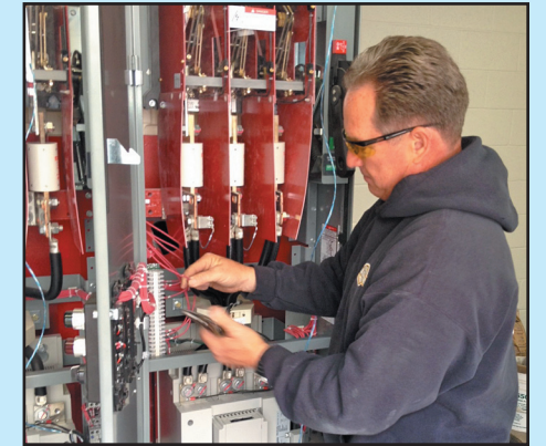
Mike Kenney with Oilfield Electric and Motor works on Casitas' electrical circuits.
