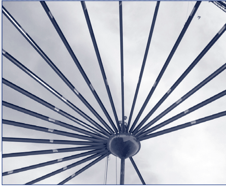
This photo depicts a worker at Casitas' Fairview reservoir tank, north of Meiners Oaks. The roof is being replaced as part of ongoing maintenance efforts.
