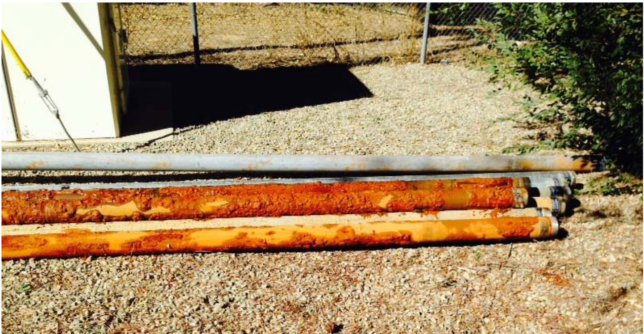
Iron Oxide Deposits on Underwater Portions of Column Pipe
