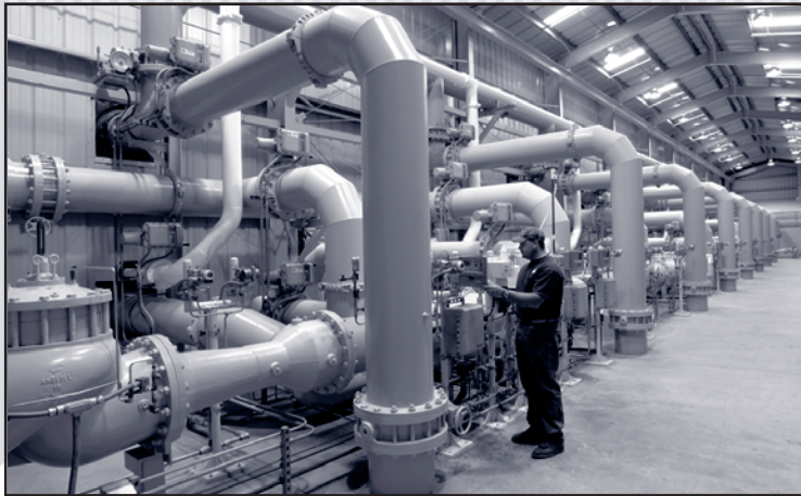
Casitas invests extensively to maintain its infrastructure. For example, Casitas recently replaced many of its aging pumps and upgraded its pumping facilities at a cost of more than $2 million.
