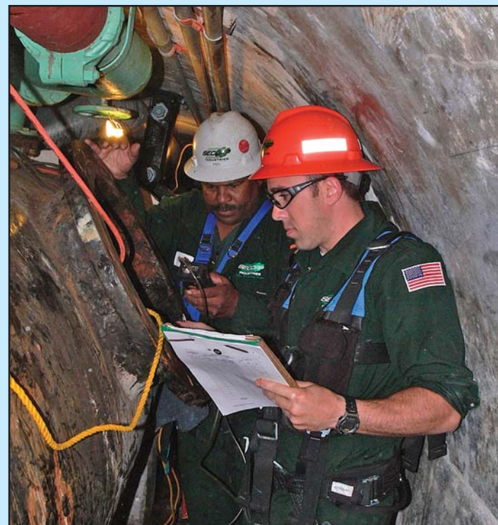
Employees from an outside contractor measure oxygen content prior to entering a confined space during a recent water inlet works inspection at Casitas Dam.
