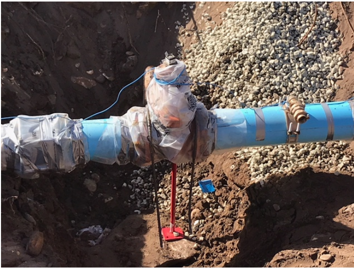
Connection Point with Isolation Valve
