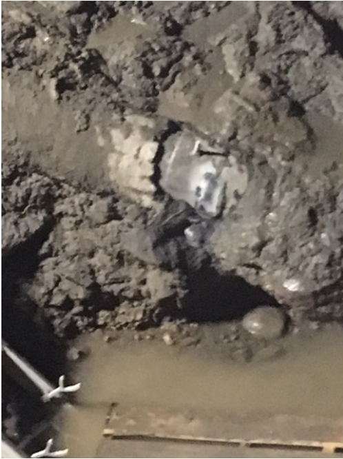
Point of Leak with Repair (Original 10" Steel Pipe)
